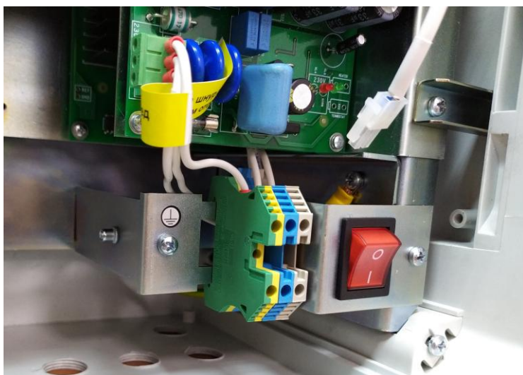
Figure 3.5.1 – Power supply unit.
